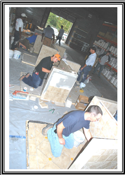
Installers are finishing up their test modules before cleaning up to take the written exam.
